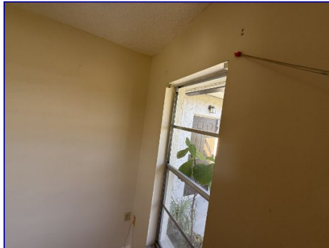
Missing all treatment and blinds
