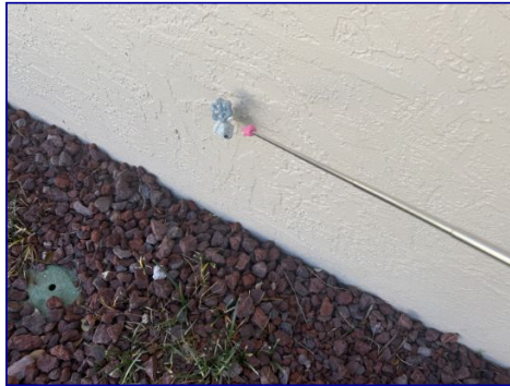
Not Functional and Capped SW corner
