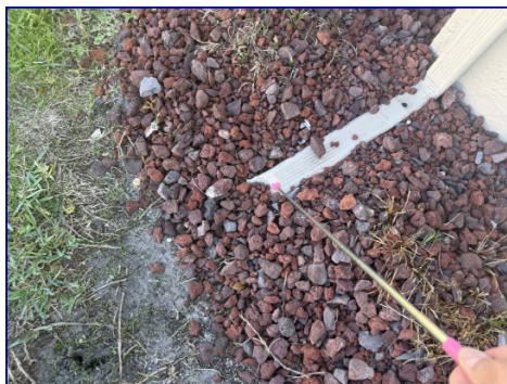
Damage on down spout NW Corner
