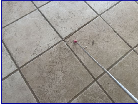
Floor grout missing and cracking
