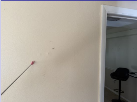
Screw Hole on Walls
