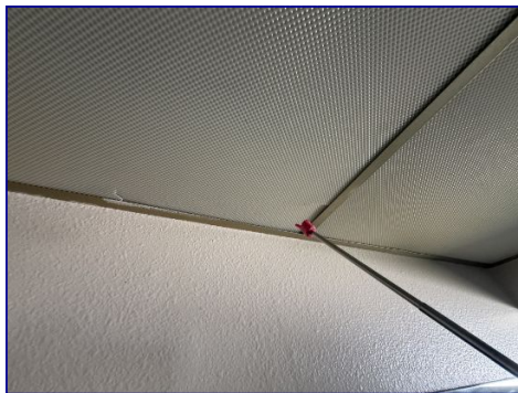
Broken over head light panel
