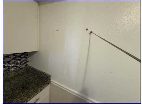
Several Bolt Holes
