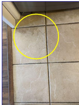
Major Cracking on Tile new Frig
