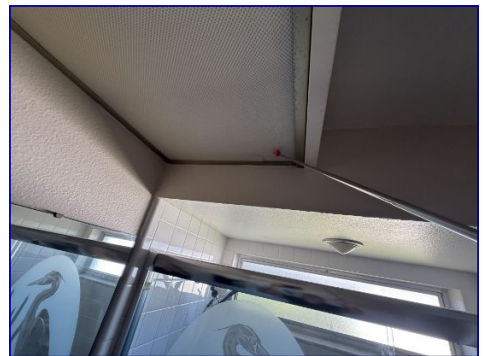
Broken over head light panel
