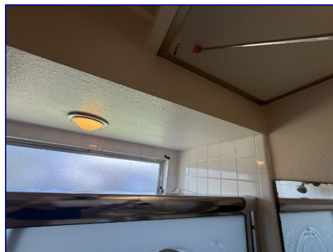
Broken Light Panel
