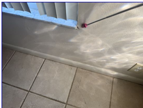
Signs of leaking
