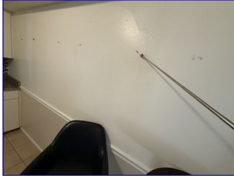
Several Bolt Holes
