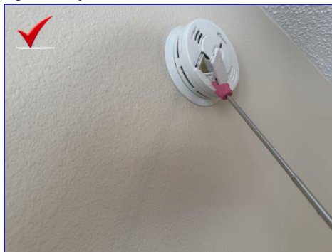
Smoke Alarm missing battery
